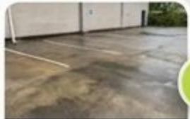
Stained Concrete Car Park
